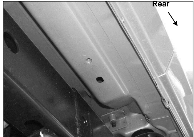
(Fig 2) Example of 2010-13 "closed" floor panel with threaded hole-10mm Nut Plate not required
